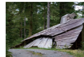
Builders of the Pacific Coast pages 98-99 Woodshed made of split cedar by Peter Buckland at Cougar Annie's (temperate rainforest field studies centre in an area named after a former inhabitant who was a legendary pioneer lady, Ada Annie Rae Arthur), British Columbia, Canada
